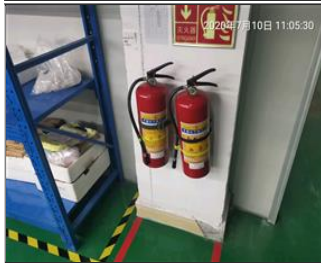
Photo of fire safety equipment fire extinguishers.jpg
