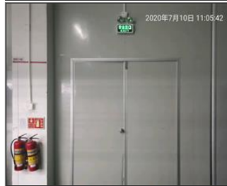
Photo of fire safety equipment exit with exit sign and emergency light.jpg
