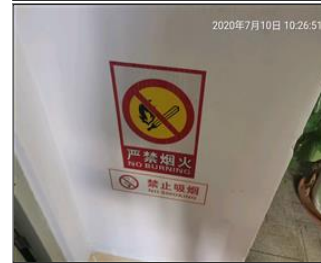
Photo of fire safety equipment no smoking sign.jpg
