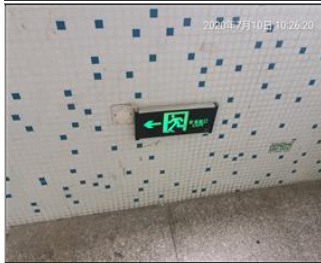
Photo of fire safety equipment evacuation route mark.jpg
