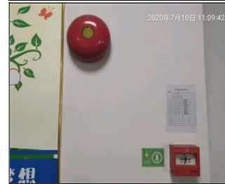
Photo of fire safety equipment fire alarm.jpg
