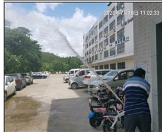
Photo of fire safety equipment test of fire hydrant.jpg
