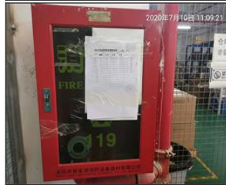
Photo of fire safety equipment fire hydrant.jpg
