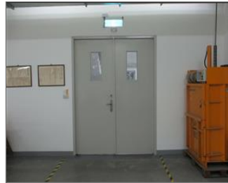
Photo of fire safety equipment Emergency exit.jpg
