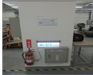
Photo of fire safety equipment Fire extinguisher.jpg
