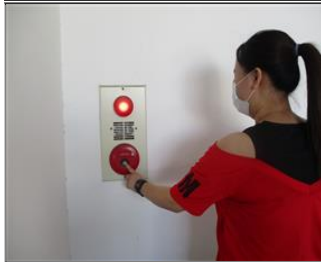
Photo of fire safety equipment Fire Alarm Being Tested.jpg
