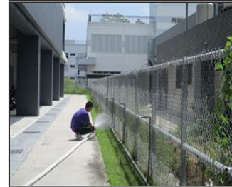
Photo of fire safety equipment Fire Hydrant Being Tested.jpg
