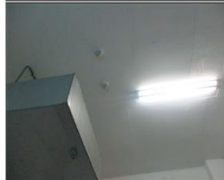
Photo of fire safety equipment Smoke Detector.jpg
