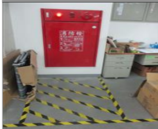
Photo of fire safety equipment Hydrant.jpg
