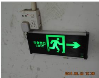
Photo of fire safety equipment Evacuation sign.JPG
