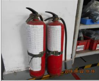
Photo of fire safety equipment Fire extinguishers.JPG
