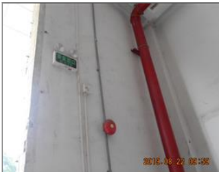
Photo of fire safety equipment Emergency light and exit sign and fire alarm.JPG
