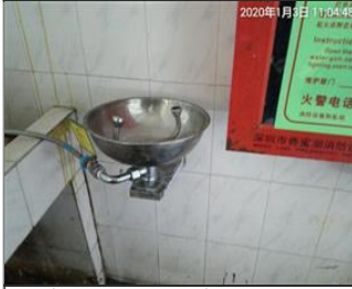
Photo of chemical storage room (if applicable) eye wash equipment.jpg
