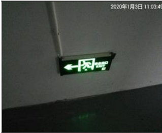
Photo of fire safety equipment evacuation indicator.jpg
