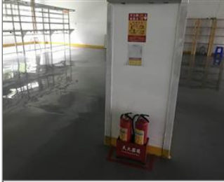
Photo of fire safety equipment Fire extinguishers.JPG
