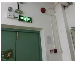
Photo of fire safety equipment Fire alarm.JPG
