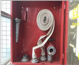
Photo of fire safety equipment Fire hydrant.JPG
