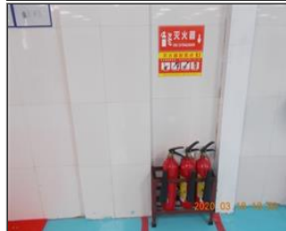
Photo of fire safety equipment Fire extinguishers.JPG
