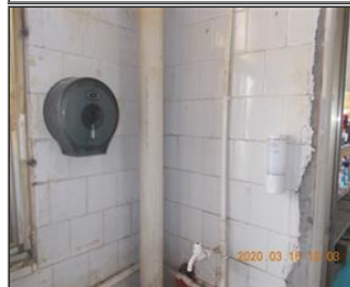
Photo of the sanitary facilities Paper and washing liquid in toilet.JPG
