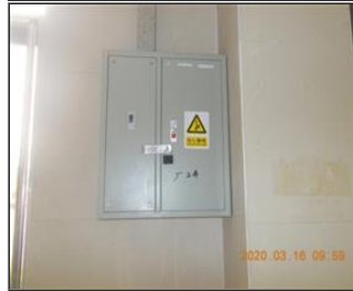
Photo of the inside of the main production hall Electricity box.JPG
