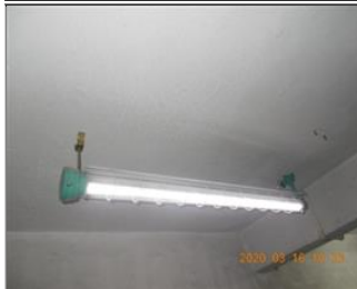
Photo of fire safety equipment Explosion-proof light.JPG
