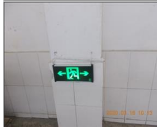
Photo of fire safety equipment Evacuation direction sign.JPG
