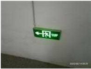
Evacuation route sign.jpg
