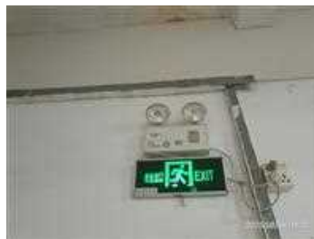
Emergency light and exit sign.jpg
