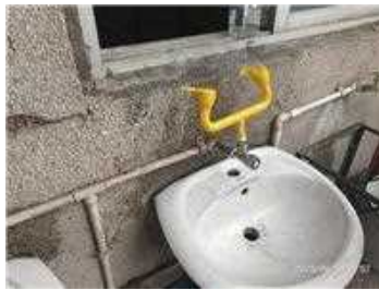
Eye wash equipment.jpg
