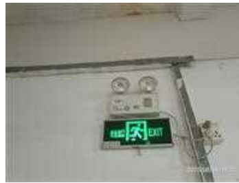
Emergency light and exit sign.jpg
