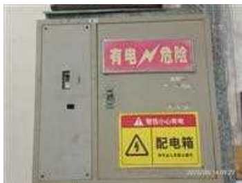
Electronic box with warning sign.jpg
