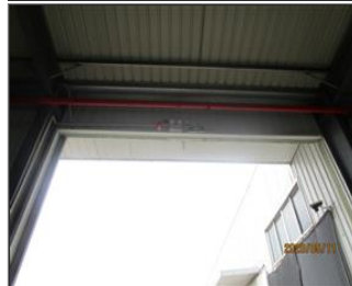
Photo of fire safety equipment fire exit sign and emergency light and fire alarm.JPG
