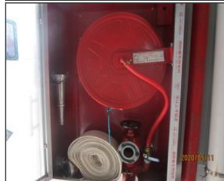
Photo of fire safety equipment fire hydrant.JPG
