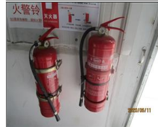
Photo of fire safety equipment fire extinguishers.JPG
