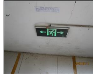
Photo of fire safety equipment evacuation direction sign.JPG
