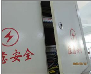
External photo(s) of the production unit(s) NC 7.13 Electric switch box without inner insulation device and not locked.JPG
