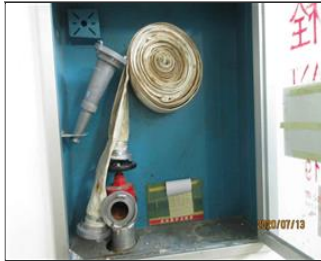
External photo(s) of the production unit(s) Fire hydrant box.JPG
