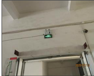
External photo(s) of the production unit(s) Exit sign and emergency light and fire alarm.JPG
