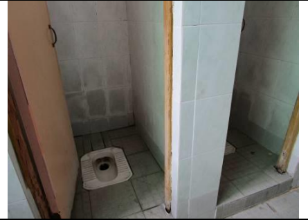
Image 42: No toilet paper and trash bins were provided to workers in the toilets of the 4-storey production building.
