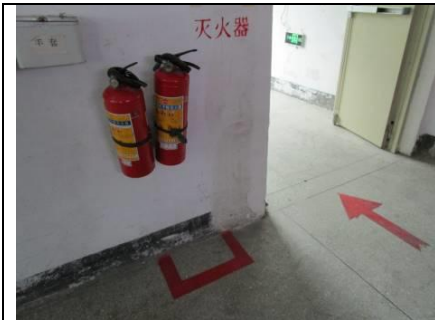
Image 13: Fire extinguishers were fully installed.
