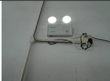
Image 10: All 2 randomly sampled emergency lights were functional when being tested.
