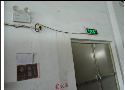
Image 9: Emergency lights and exit signs were installed above all fire exits.
