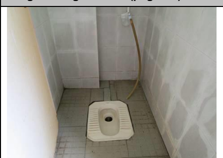
Image 36: No toilet paper and trash bins were provided to workers in the toilets of the dormitory building.
