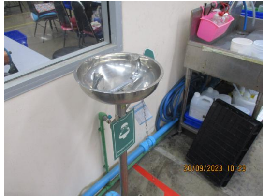
Eye Wash Station.JPG
