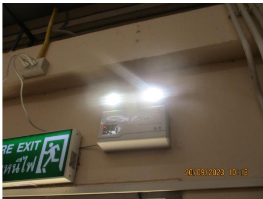
Emergency Light Testing.JPG
