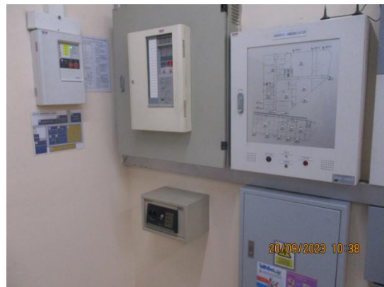
Fire Alarm Control Panel.JPG
