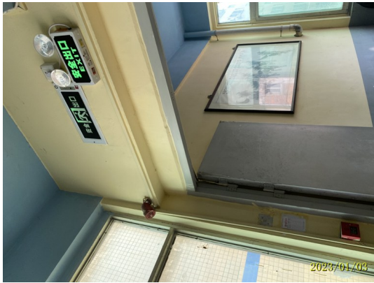
Fire alarm, safety exit sign and emergency light.JPG
