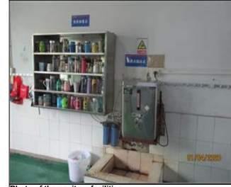
Photo of the sanitary facilities drinking water.JPG
