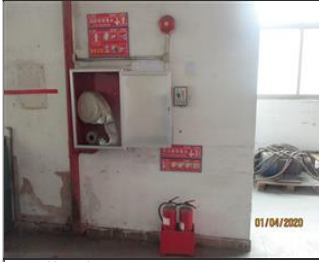
Photo of fire safety equipment fire alarm and fire hydrant and fire extinguishers.JPG
