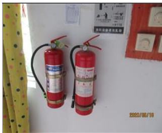
Photo of fire safety equipment Fire extinguishers.JPG
