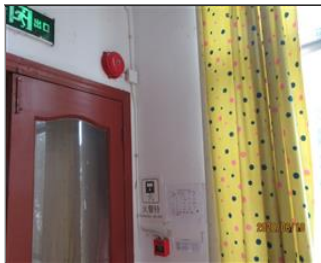
Photo of fire safety equipment Fire alarm.JPG
