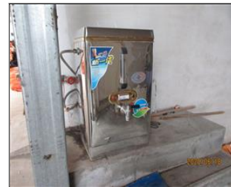
Photo of the sanitary facilities Potable water.JPG
