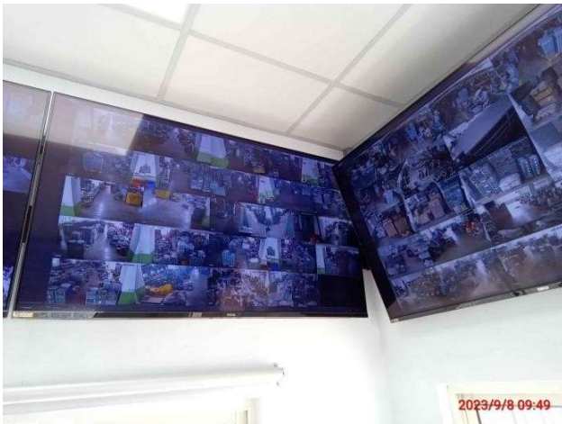
CCTV system and monitor
