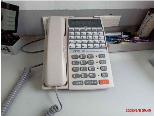
Security Room – Communication Equipment
