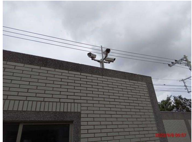
CCTV system and monitor
