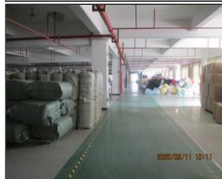
Photo of fire safety equipment Fire sprinkler in warehouse.JPG
