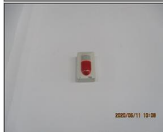
Photo of fire safety equipment Fire alarm.JPG
