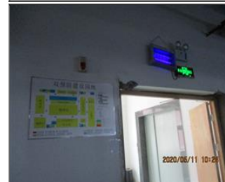
Photo of fire safety equipment Safety exit sign and emergency light and fire alarm.JPG
