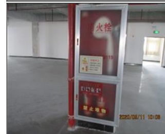
Photo of fire safety equipment Fire facility.JPG
