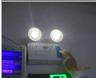
Photo of fire safety equipment Test of emergency light.JPG
