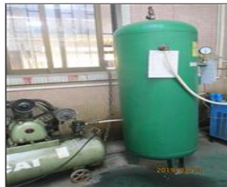
Photo of the inside of the main production hall Air tank.JPG
