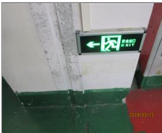
Photo of fire safety equipment Evacuation sign.JPG
