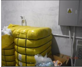
External photo(s) of the production unit(s) 7.13 Flammable laid beside electric box.JPG
