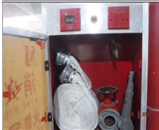
External photo(s) of the production unit(s) Fire hydrant and fire alarm.JPG
