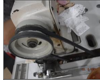
External photo(s) of the production unit(s) 7.17 Without pulley guard.JPG
