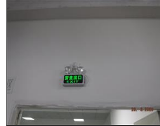
External photo(s) of the production unit(s) Safety exit sign and emergency light.JPG
