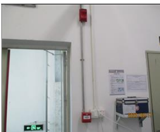
Photo of fire safety equipment Fire Alarm.JPG
