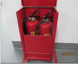
Photo of fire safety equipment Fire Extinguisher.JPG
