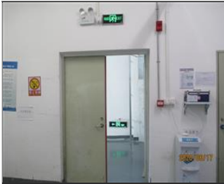
Photo of fire safety equipment Emergency Light and Exit.JPG
