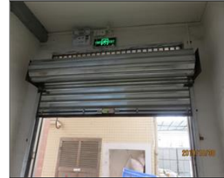
Photo of fire safety equipment emergency exit and emergency light.JPG
