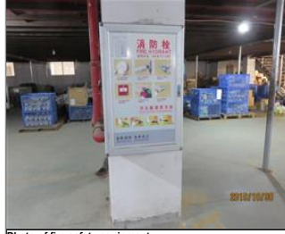
Photo of fire safety equipment fire hydrant.JPG
