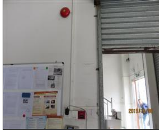
Photo of fire safety equipment fire alarm.JPG
