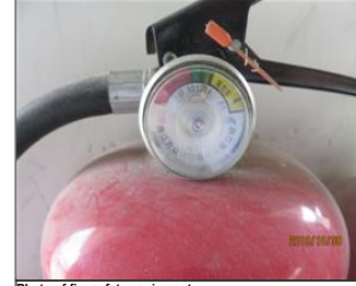
Photo of fire safety equipment sufficient pressure of fire extinguisher.JPG
