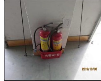
Photo of fire safety equipment fire extinguishers.JPG
