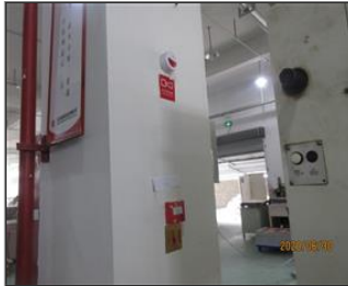
Photo of fire safety equipment 4-2 Fire alarm.JPG
