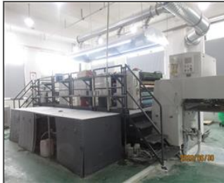
Photo of the inside of the main production hall 9-1 printing.JPG
