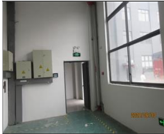
Photo of fire safety equipment 4-4 Emergency lamp and Exit sign.JPG
