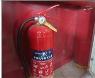
Photo of fire safety equipment 4-1 Fire extinguisher.JPG
