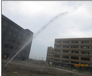
Photo of fire safety equipment 4-5 Test of fire hydrant.JPG
