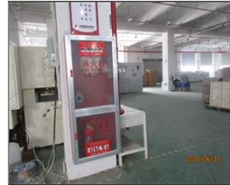
Photo of fire safety equipment 4-3 Fire hydrant.JPG
