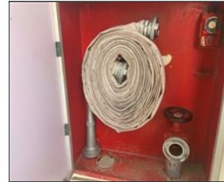
External photo(s) of the production unit(s) Hydrant.JPG
