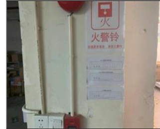
External photo(s) of the production unit(s) Fire alarm.JPG
