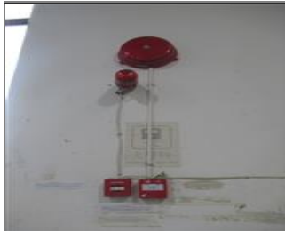
Photo of fire safety equipment Fire alarm.JPG
