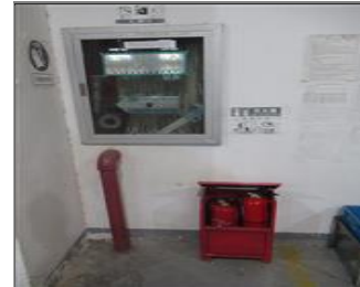
Photo of fire safety equipment Fire hydrant and fire extinguishers.JPG
