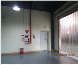
Photo of fire safety equipment Emergency light Exit mark Evacuation plan Hydrant Fire alarm Extinguishers.JPG
