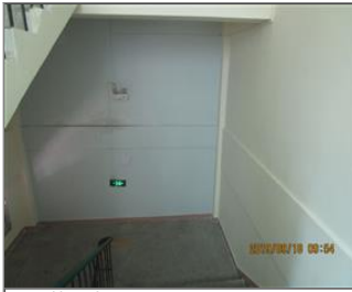
Photo of fire safety equipment Emergency light Evacuation indicating sign in the staircase of the workshop.JPG
