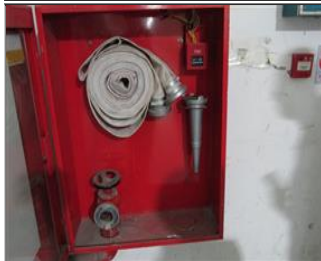
Photo of fire safety equipment Fire hydrant.JPG
