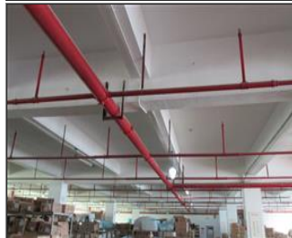
Photo of fire safety equipment Sprinkler system.JPG
