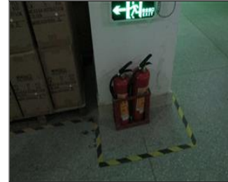
Photo of fire safety equipment Fire extinguishers.JPG
