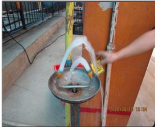
Photo first aid facilities Eye washing facility.JPG
