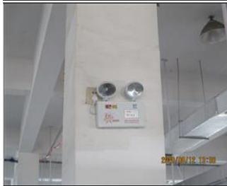
Photo of fire safety equipment Emergency light.JPG
