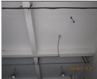
Photo of fire safety equipment Fire sprinkler system and smoke detector.JPG
