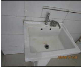
Photo of non-conformity NC-No soap and toilet paper provided in toilet.JPG
