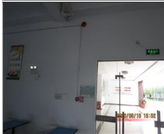
Photo of fire safety equipment Exit sign and emergency lighting testing were OK.JPG
