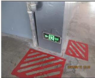
Photo of fire safety equipment Evacuation indicating sign.JPG
