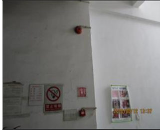
Photo of fire safety equipment Fire alarm.JPG
