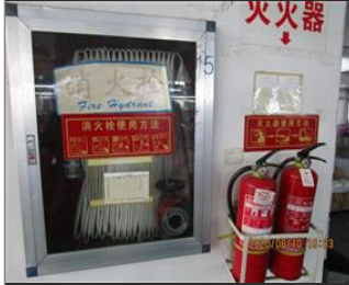
Photo of fire safety equipment Fire extinguishers and fire hydrant.JPG
