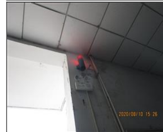
Photo of fire safety equipment Fire alarm testing was OK.JPG
