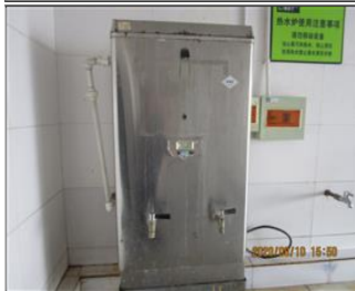
Photo of the sanitary facilities Potable water.JPG
