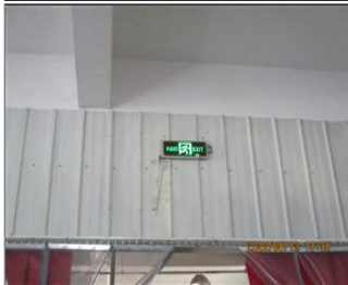
Photo of fire safety equipment Exit sign.JPG
