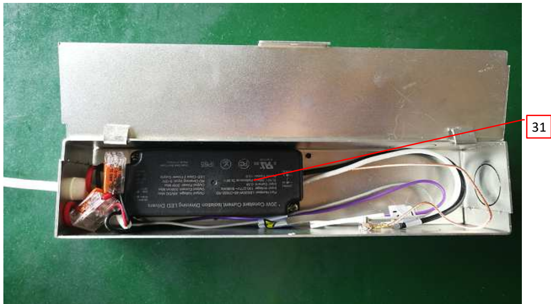
Photo 79 - Internal junction box view for VMCL000701A020, VMDL000701A020, VMCL001901C020, VMCL001901D020
