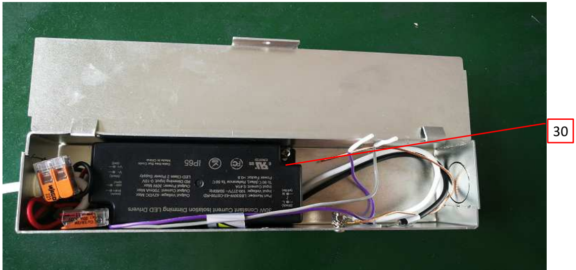
Photo 77 - Internal junction box view for VMDL000610C024, VMDL000610E024, VMDL000610A024
