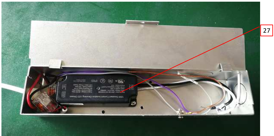
Photo 78 - Internal junction box view for VMDL000603A009, VMDL000605A012, VMDL000605E012, VMDL000603C009, VMDL000605C012, VMCL000605D012, VMCL000605E012, VMDL003001B012, VMCL001901A012, VMCL001901B012
