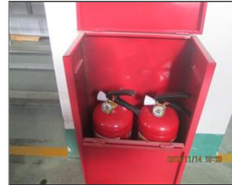
Photo of fire safety equipment Fire extinguisher.JPG
