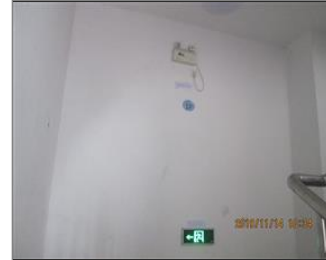
Photo of fire safety equipment Emergency lighting and evacuation sign in staircase.JPG
