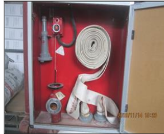
Photo of fire safety equipment Fire hydrant.JPG
