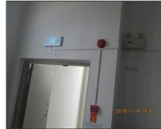
Photo of fire safety equipment Safety exit and fire alarm.JPG
