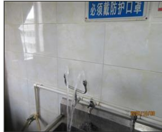
External photo(s) of the production unit(s) eye wash facility.JPG
