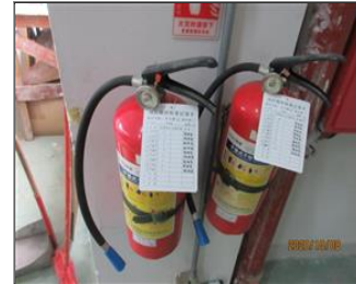
External photo(s) of the production unit(s) fire extinguishers.JPG
