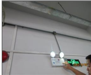
External photo(s) of the production unit(s) testing of emergency light.JPG
