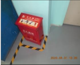
Photo of fire safety equipment Fire extinguisher.JPG
