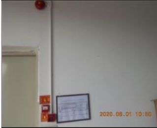
Photo of fire safety equipment Fire alarm.JPG
