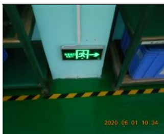
Photo of fire safety equipment Evacuation sign.JPG
