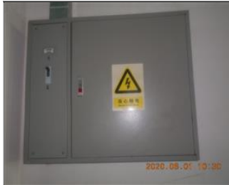
Photo of fire safety equipment Electric box.JPG
