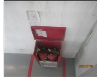
Photo of fire safety equipment Fire extinguishers.JPG
