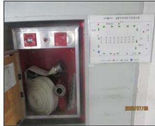
Photo of fire safety equipment Fire hydrant.JPG
