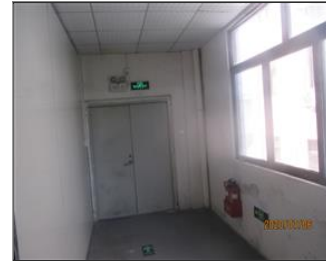
Photo of fire safety equipment Safety exit.JPG
