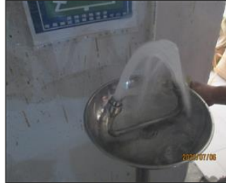
Photo first aid facilities Eye washing station.JPG
