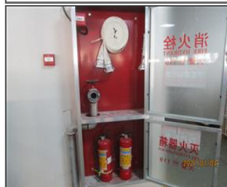
Photo of fire safety equipment Fire hydrant and fire extinguisher.JPG
