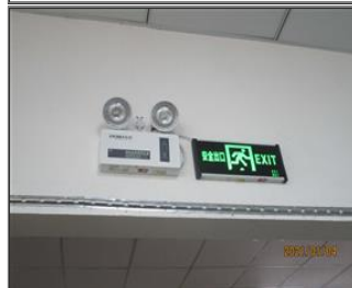
Photo of fire safety equipment Emergency light and exit sign.JPG
