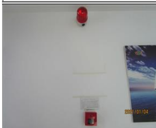
Photo of fire safety equipment Fire alarm.JPG
